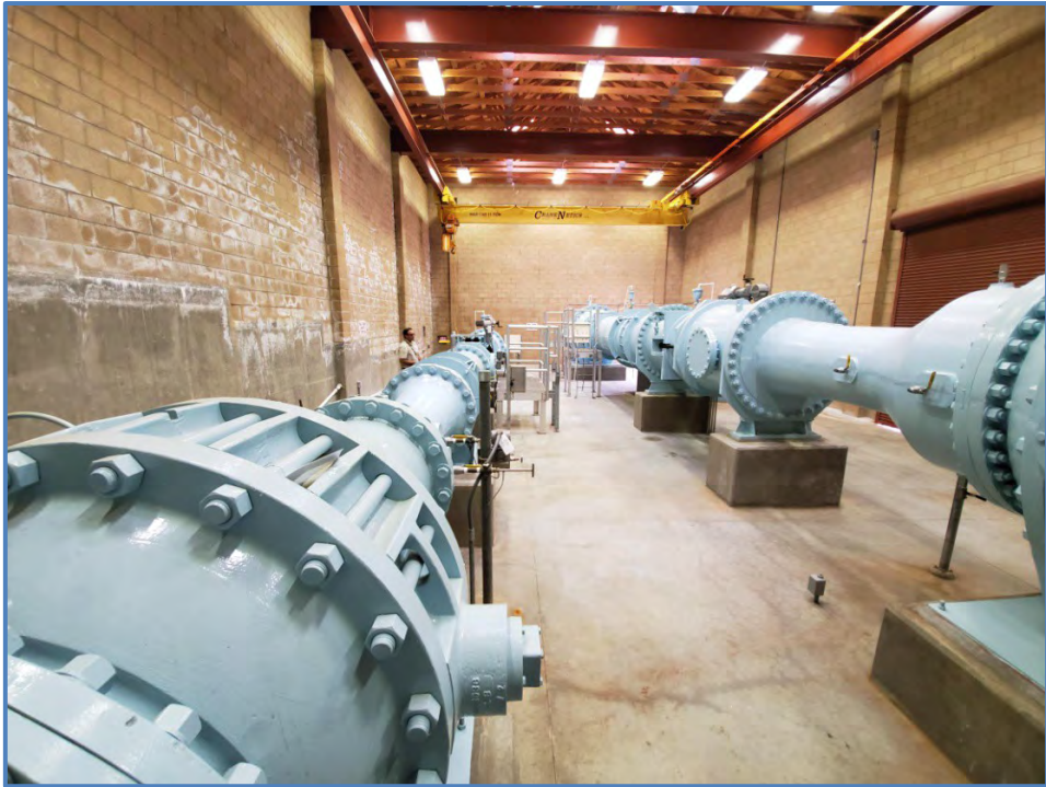
Figure 7.4 – Typical Piping, Valves and Equipment inside FCF (Large Size)
