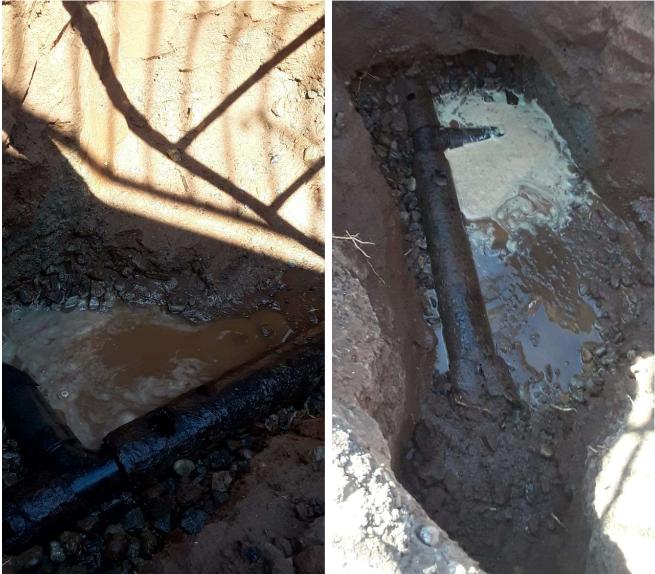
Leach lines as appears at branch, with sewage backed-up, note corroded/deteriorated pipes.
