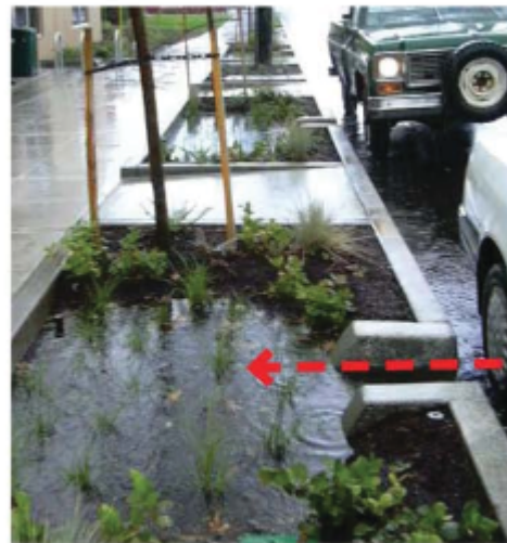
Figure 5-33: A standard curb with wings allows stormwater runoff to enter a stormwater facility. The wings help retain the side slope grade on each side of the curb cut opening.
