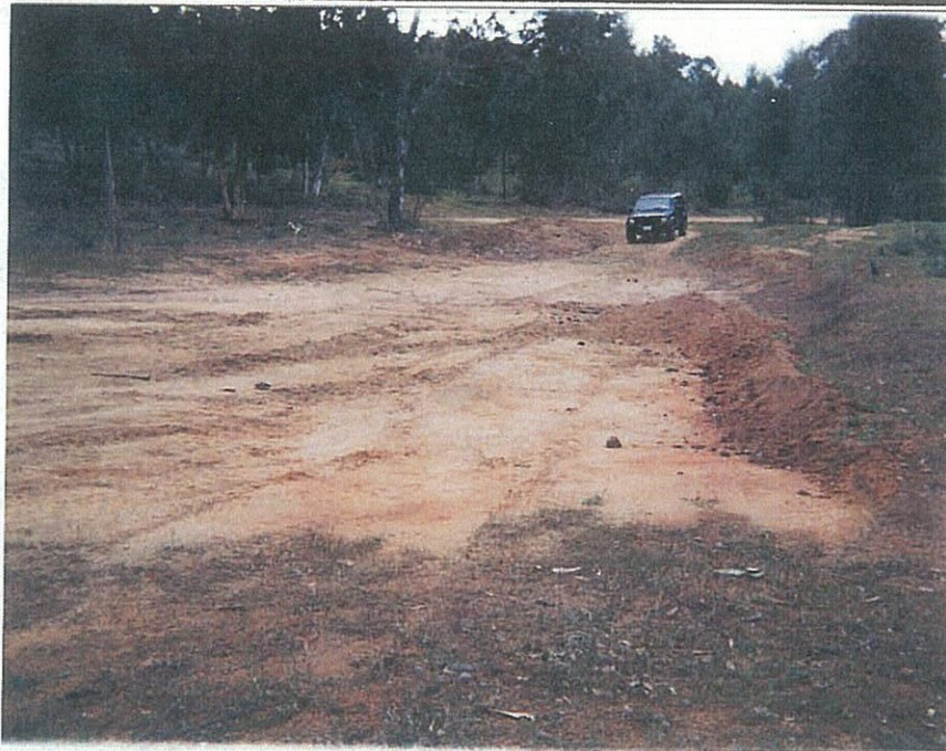
3. Excavation area in south central portion of ranch property. Area, located within rectangular tree cluster, was the previous location of the ranch dump. View is to southeast.
