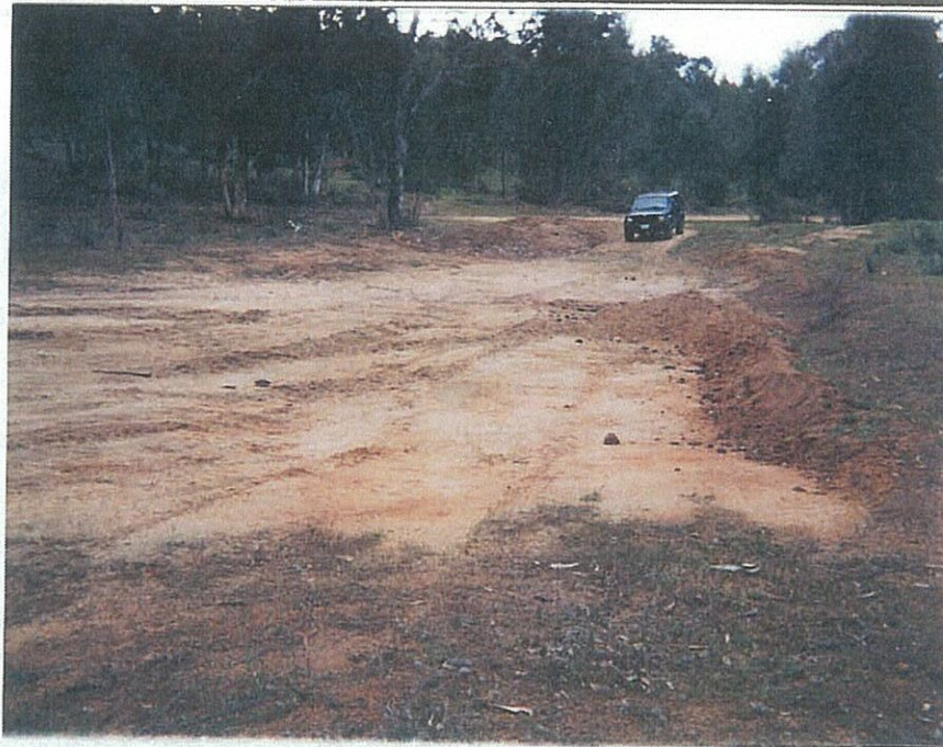
3. Excavation area in south central portion of ranch property. Area, located within rectangular tree cluster, was the previous location of the ranch dump. View is to southeast.
